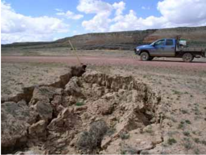
Figure 4.9-3. Example of erosion resulting from concentration of surface runoff at drainage crossings
