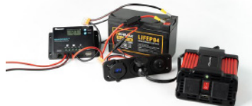
Entire 40 W PV system including a charge controller with two solar panels in parallel and a 12 V battery running an inverter. Solar panels not pictured.
