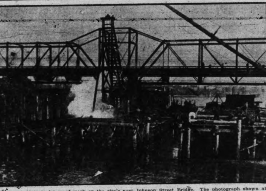
This is the latest picture of work on the city's new Johnson Street Bridge. The photograph shown above was taken by City Engineer F. M. Preston, who is supervising the installation of the new bridge foundations. It shows a large steam pile driver ramming heavy piles into the mud of the harbor bottom within one of the enormous box-like wooden caissons. Upon these piles will be built the cement bridge piers which will support the bridge superstructure.
