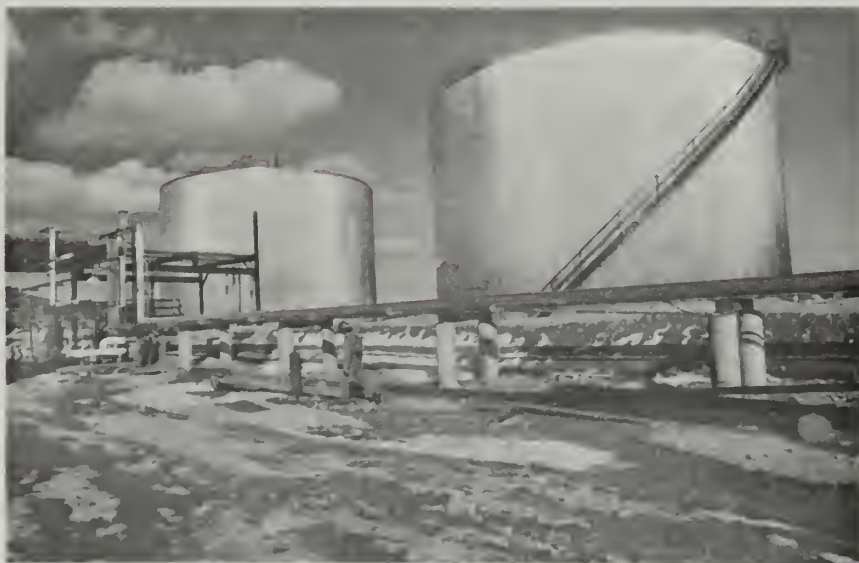
FIGURE 6-5-1 RETORT OIL AND SOUR WATER STORAGE TANKS
