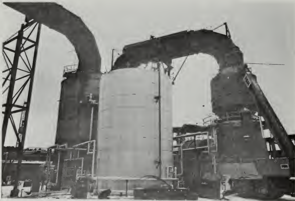
FIGURE 3-2-15 SODA ASH STORAGE TANK (FOREGROUND)
