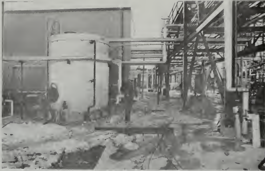
FIGURE 3-2-14 PROCESSING PLANT PIPE RACK AND CONDENSATE COLLECTION TANK
