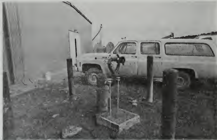
FIGURE 6-3-1 FIRE HYDRANT AND TURRET NOZZLE - PROCESSING PLANT AREA
