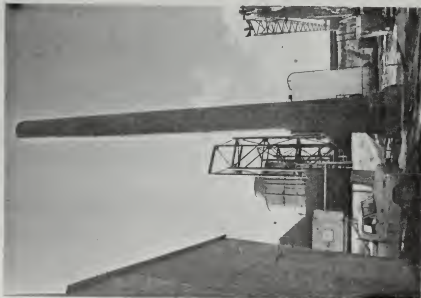
FIGURE 3-2-10 STEAM GENERATOR BOILER STACK
