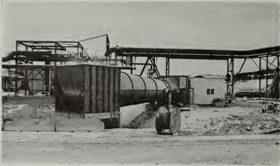
FIGURE 2-3-5 MAIN MINE VENTILATION FAN
