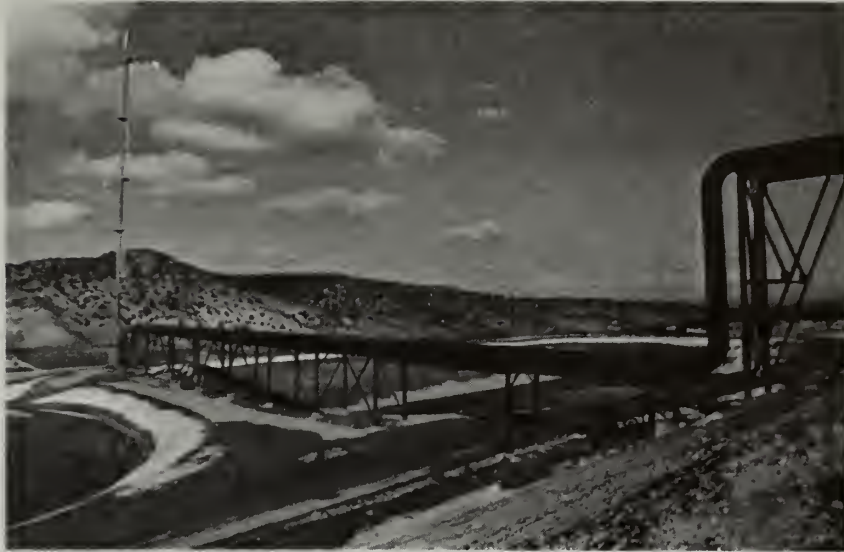
FIGURE 3-2-8 ELEVATED PIPELINE AND EMERGENCY FLARE STACK
