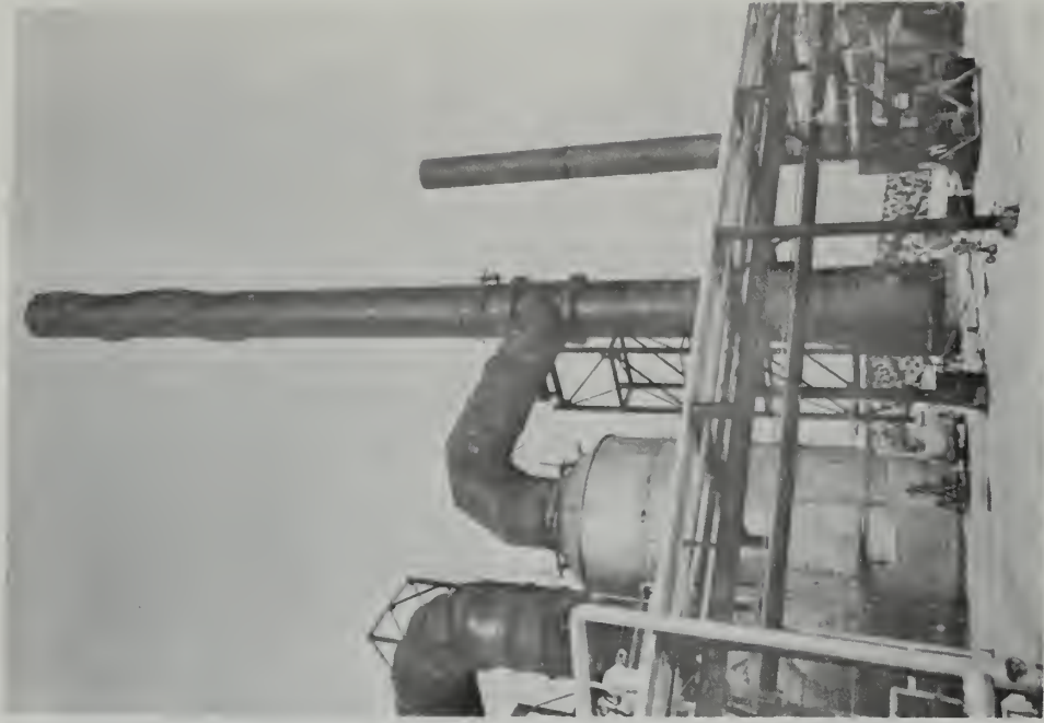
FIGURE 3-2-7 200 FT. SCRUBBER STACK (CENTER)
