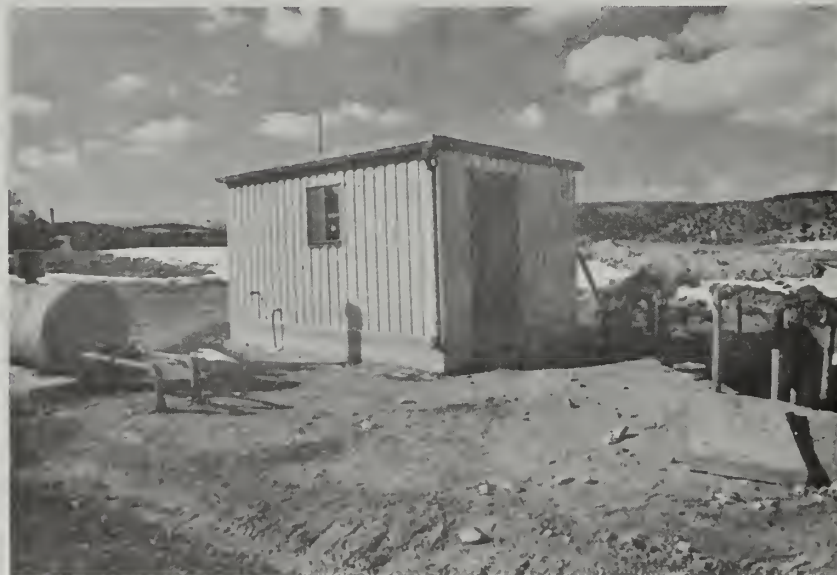
FIGURE 5-2-1 NATURAL GAS METERING STATION
