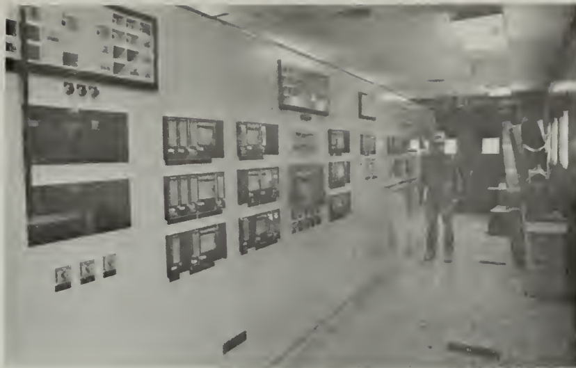
FIGURE 3-2-16 PROCESSING PLANT CONTROL ROOM
