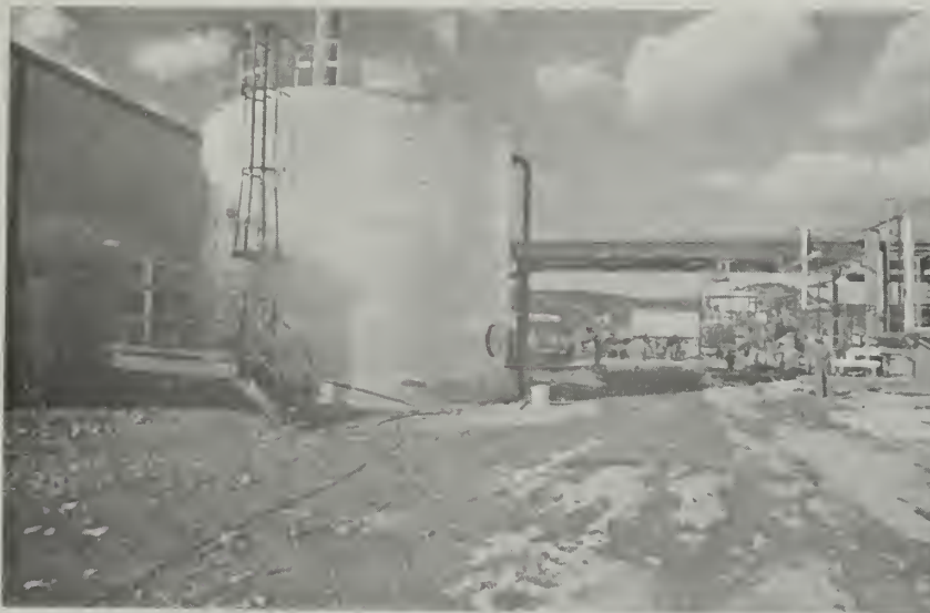
FIGURE 3-2-13 BOILER FEEDWATER STORAGE TANK
