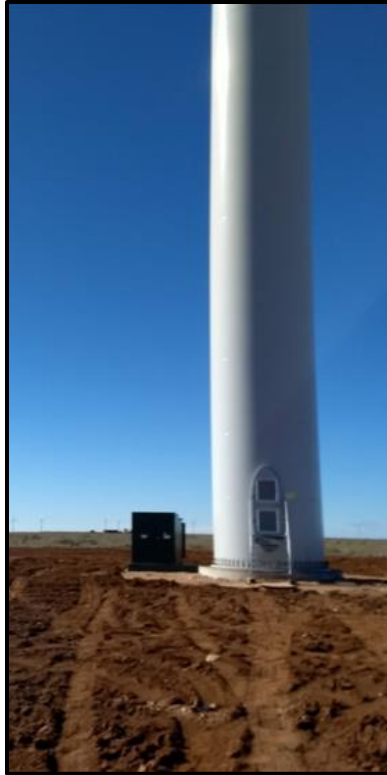
Figure 8. Typical pad-mounted transformer.
