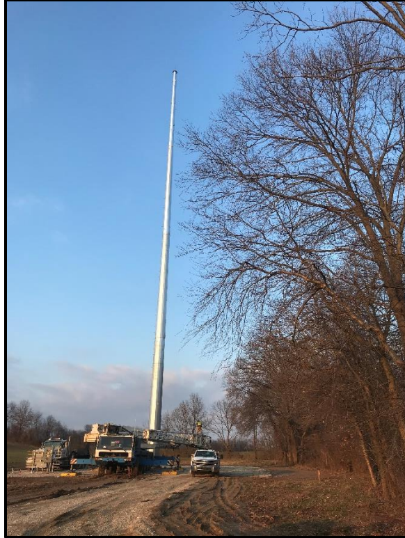
Figure 16. Typical monopole meteorological tower.
