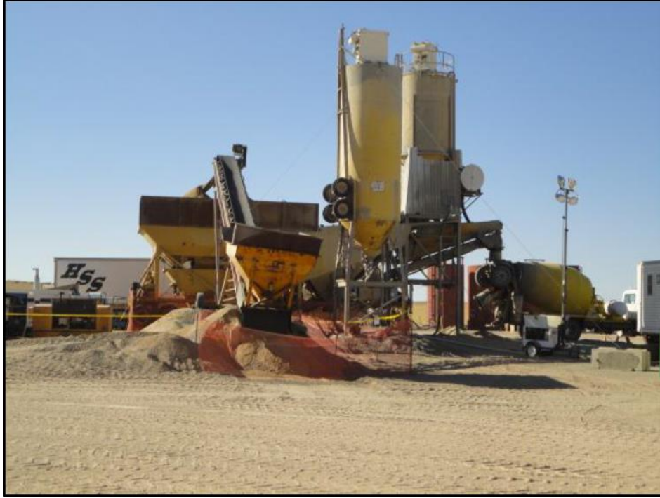
Figure 18. Typical temporary concrete batch plant.
