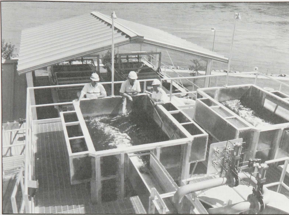
Volunteer workers at the new Little Goose juvenile fish bypass facilities during the first season of operation, June 1990.
