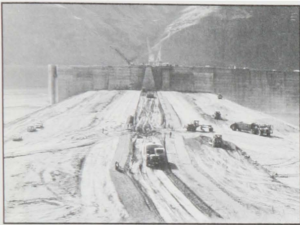
Earth mover heading for the earth fill part of Lower Granite Dam, October 1974.
