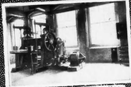
15-h.p., 600-r.p.m., 550-volt Slip Ring Induction Motor and Panel for Plaster
