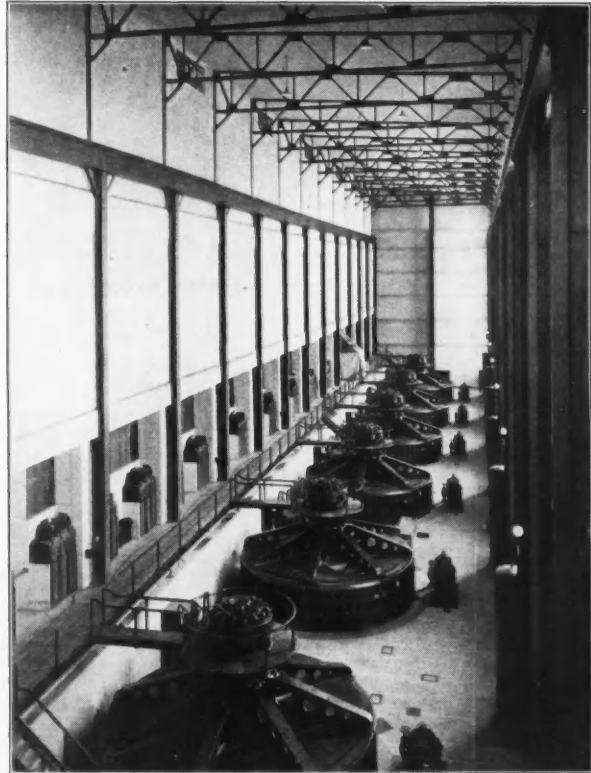
The governor for each unit is driven by a lay shaft geared to the main turbine shaft. Water is supplied under 200 lb. pres-
