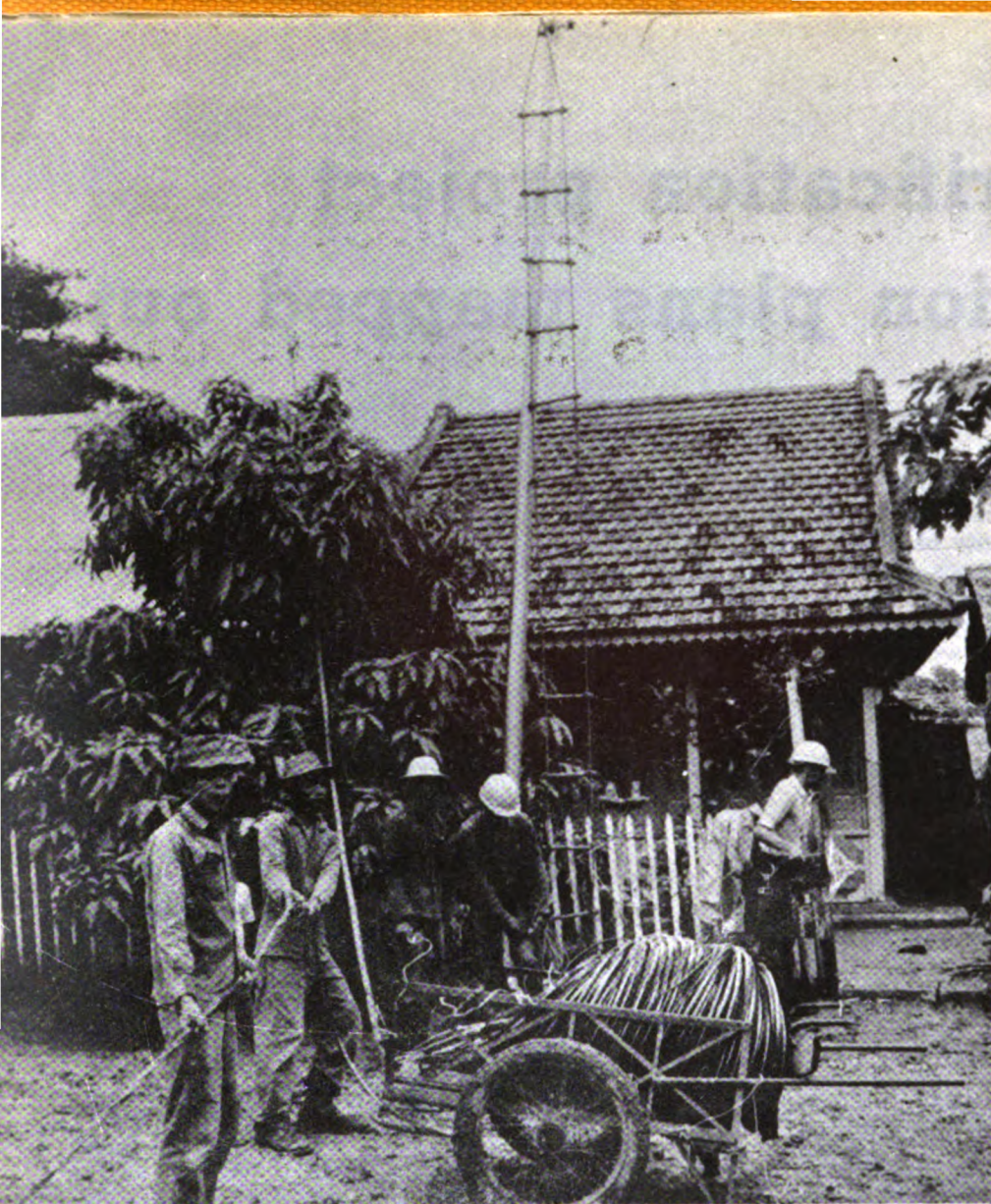
This wire is bringing electricity to an An Giang home that was lighted by oil lamps before the province's rural electric cooperative was formed.
