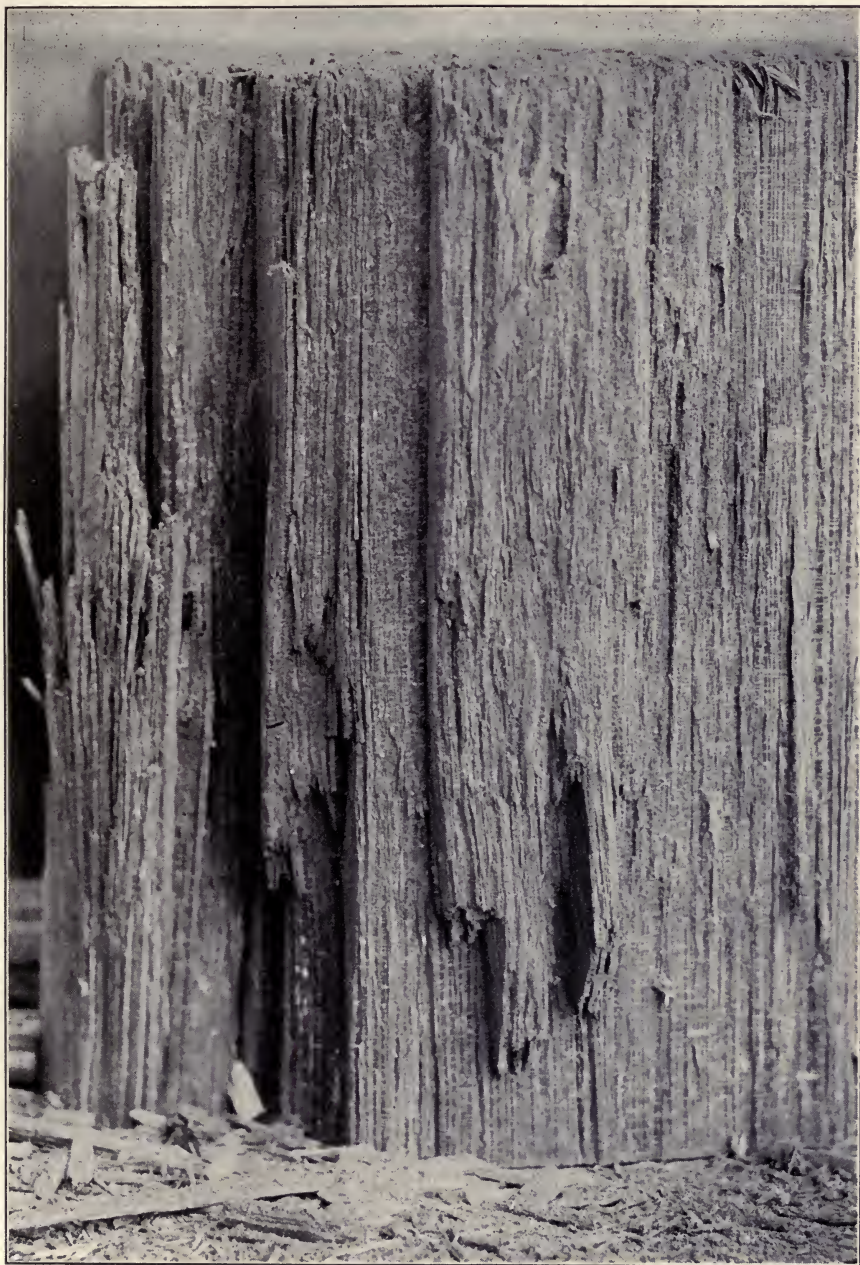
Lifeless Condition of Wood is Shown by Detached Material at Bottom of Picture.
