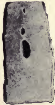
FIG. 62.—Perforation in sheet-lead roof made by adult beetle.
