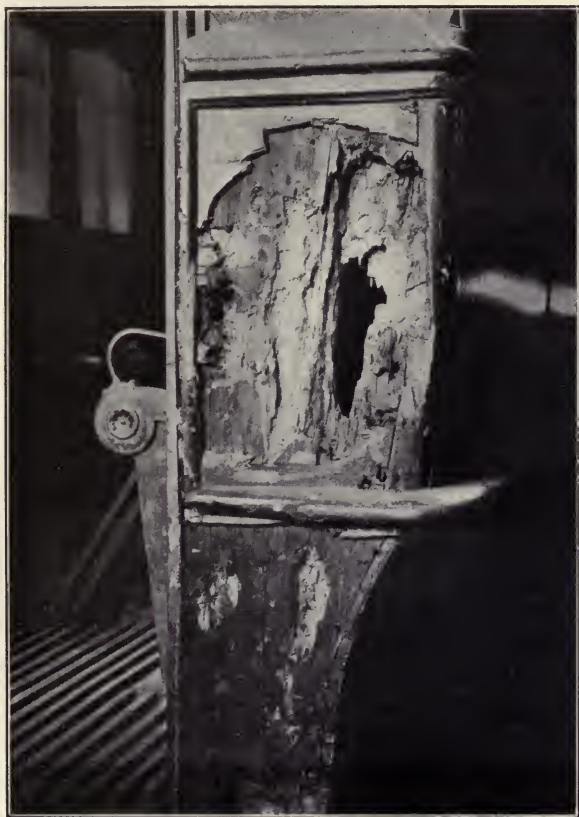
FIG. 79.—Failure of car post due to application of paint upon imperfectly seasoned wood.
