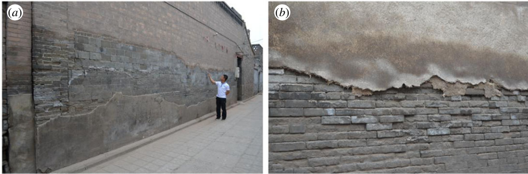
Figure 11. The practice of (a) smearing cement or (b) clay and plant fibres on the ancient brick in walls failed to prevent weathering of the ancient bricks.
