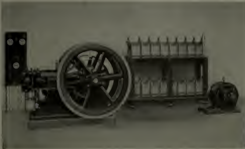
A complete low voltage electric plant for the country home, showing engine, generator, switchboard, and a small storage battery of sixteen cells
