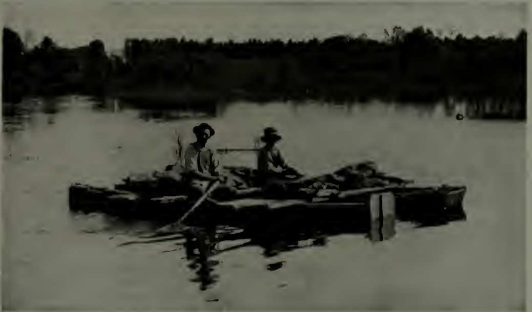
Hauling stone for the foundation. The boats were lashed together side by side, and planks laid across them. The boatmen rowed backward in order to see better when making the landing
