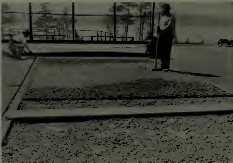
Tamping and leveling the court. The section to the right has been screeded and is now complete except for grading and rolling
