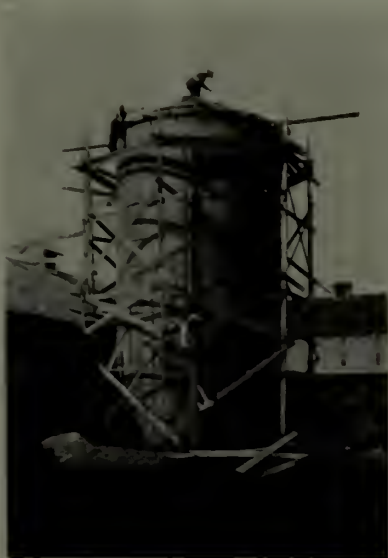
A stave silo in process of construction, showing the scaffolding still up
