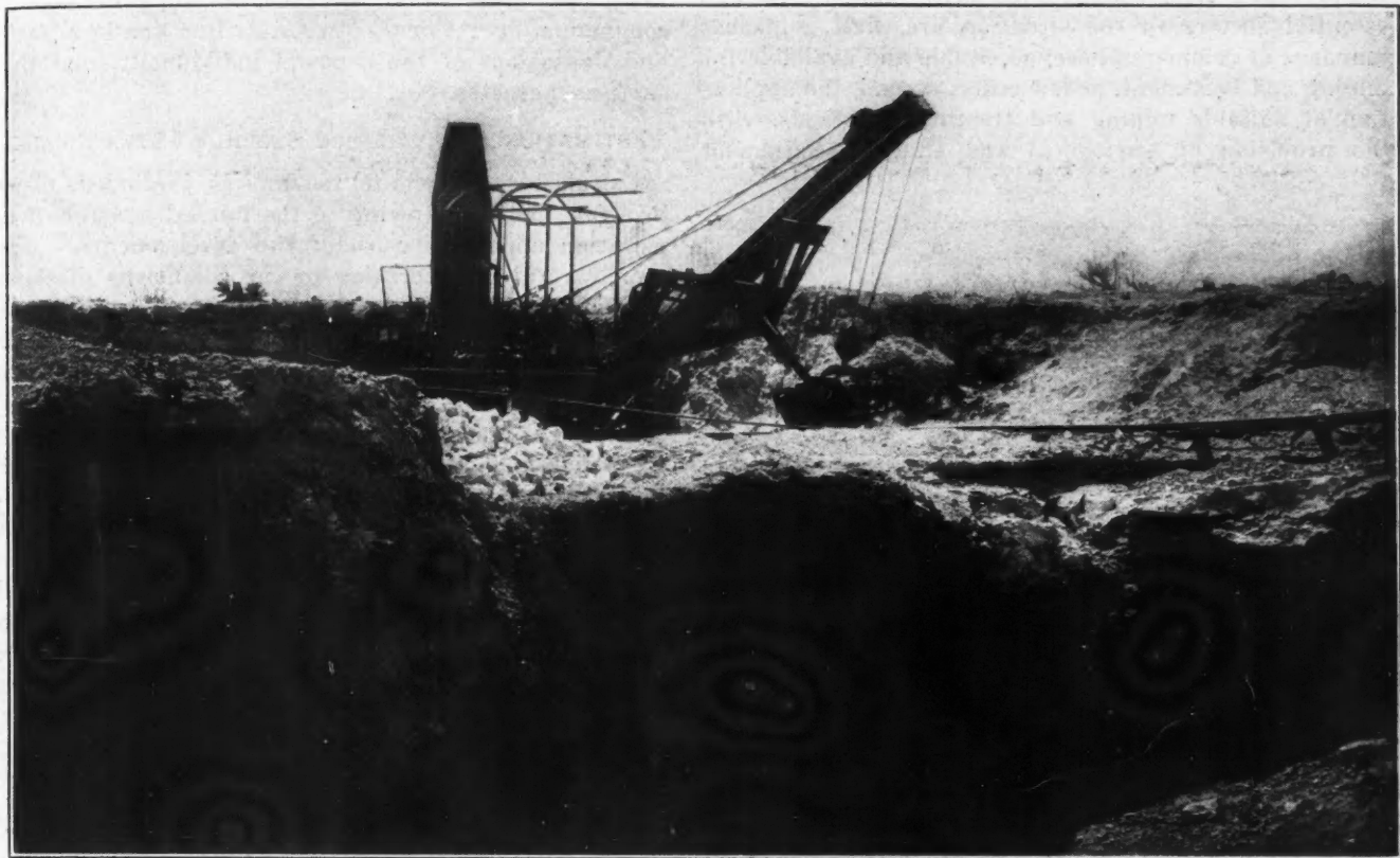
FIG. 1. STEAM SHOVEL OPERATING IN THE OREBODY OF THE WEST TEXAS SULPHUR COMPANY
