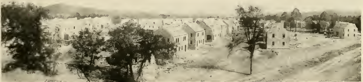
U. S. Housing Project No. 18, South Charlestown, West Virginia. Picture taken at time buildings were being constructed. Every house is built of Hollow Tile and finished with stucco.
