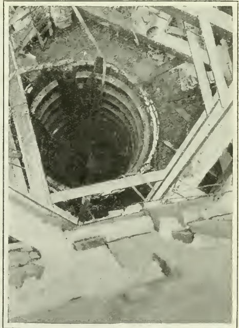
No. 1 Caisson, No. 2 Pier, 8 inches from Rock. Michigan Central Railway Bridge—Montrose. Nov. 10, 1921
