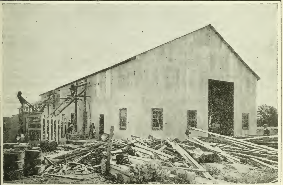
Montrose Substation Rebuilt: Eight and a Half Days after Destruction of Original Substation by Fire
