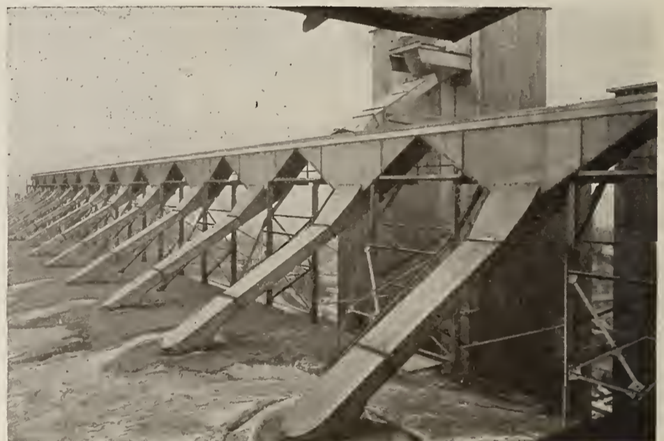
V-SPOUTS WHICH RECEIVE GRAIN FROM THE MARINE TOWER LOFTER LEGS
