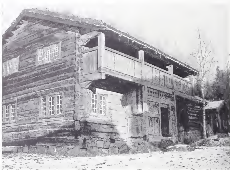
MAIHAUGEN OPEN-AIR MUSEUM: ONE OF THE BJÖRNSTAD CLUSTER OF HOUSES NOW IN COURSE OF ERECTION
