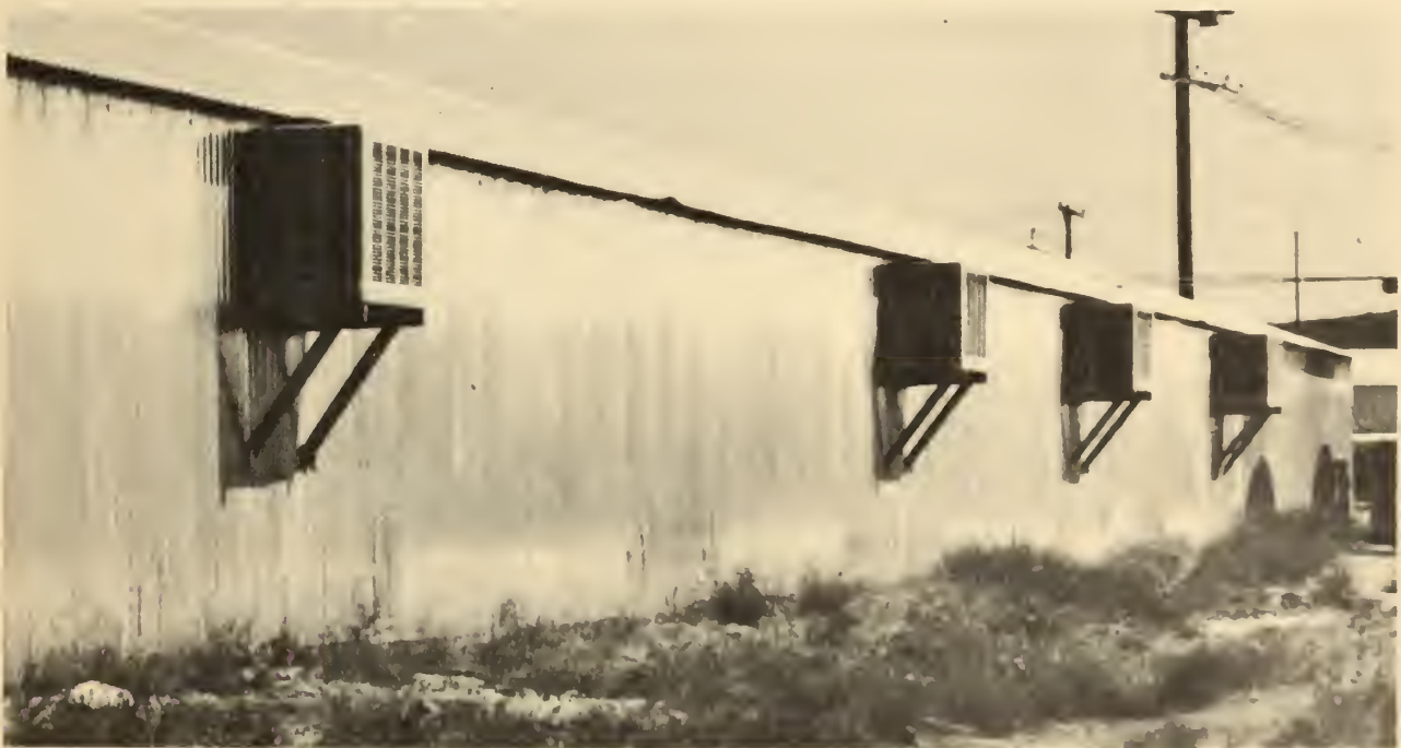
FIGURE 14.—Windowless laying house in southern California with packaged window-type evaporative coolers in sidewalls.
