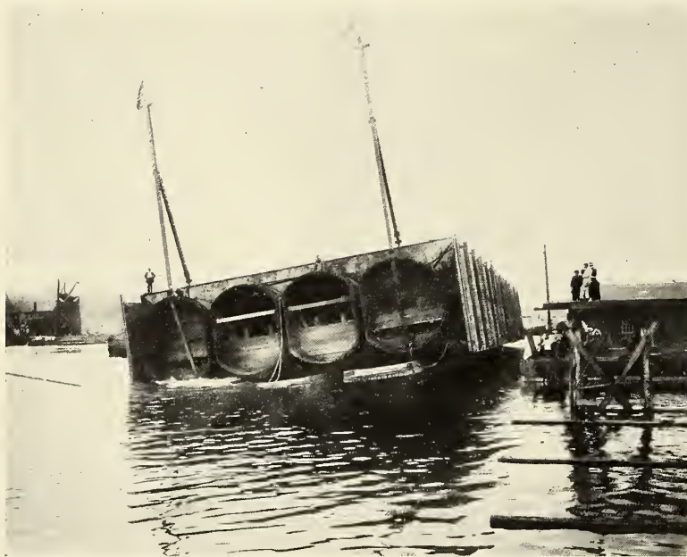
LAUNCH OF THE TUNNEL SECTION. PHOTOGRAPH TAKEN JUST AS ONE OF THE FLATBOATS HAD SUNK AND THE SECTION WAS LURCHING TO THAT SIDE.
