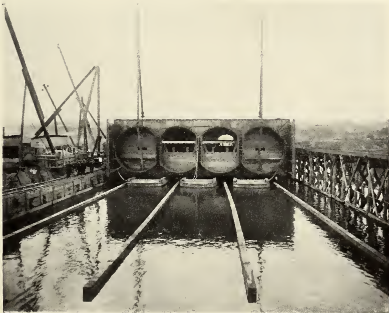
LIFTING A TUNNEL SECTION OFF THE STAGING ON WHICH IT WAS BUILT, BY MEANS OF FLATBOATS RAISED BY THE TIDE.
