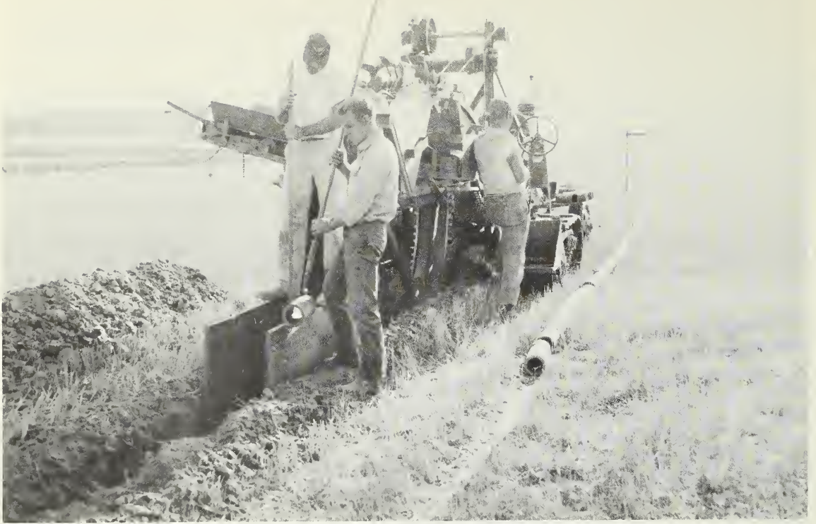
Sighting bar used to maintain grade on wheel trench excavator. Four-inch clay tile is being placed by hand. Soil is suitable for blinding, filter and backfill. (Photo No. 0-883-11)
