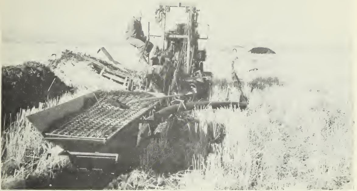
Plastic tubing installed as an interceptor with crushed, light-weight basaltic tuff as bedding and envelope material. (Photo No. 0-3057-14)
