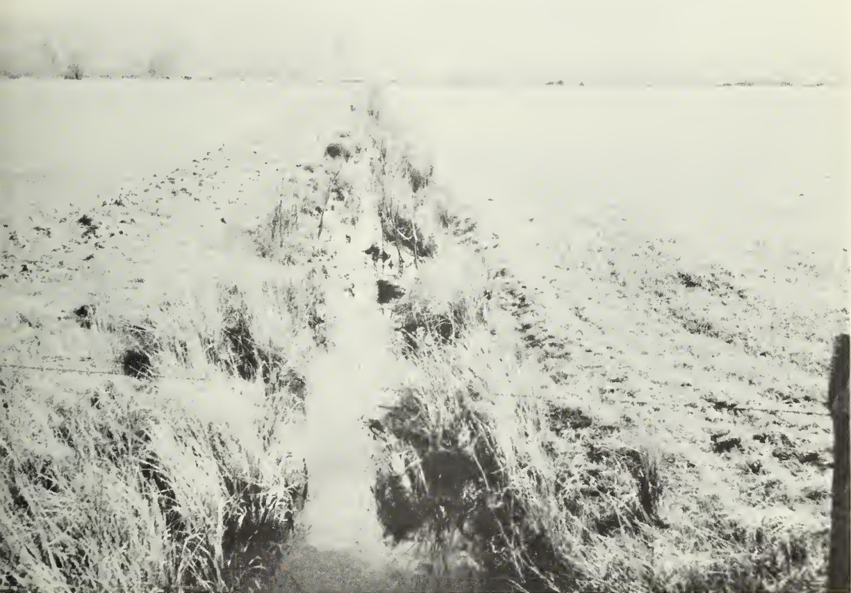
Drainage ditch in need of maintenance work. (Photo No. 0-1220-7)
