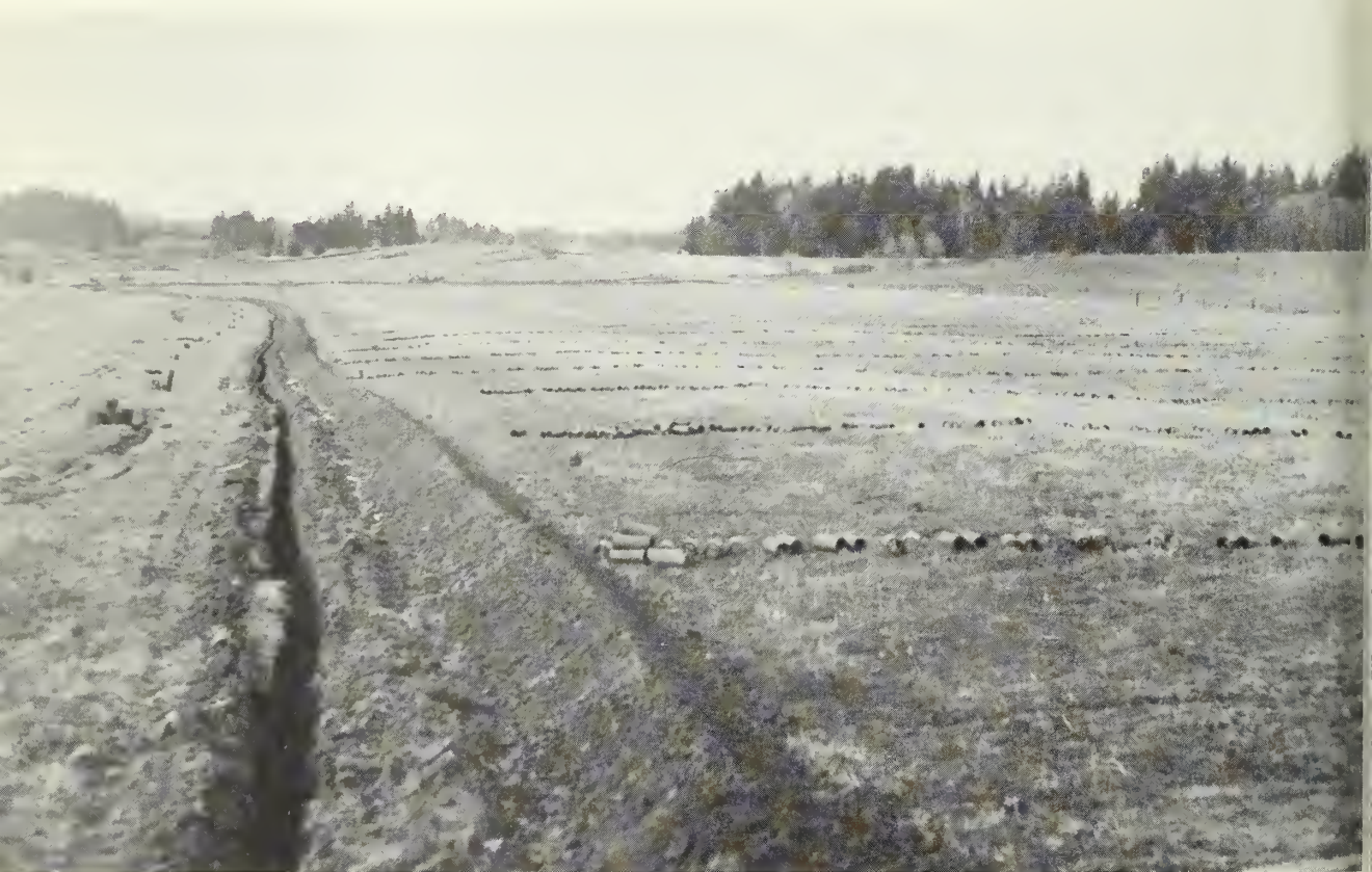
Clay tile being installed in a parallel pattern. Outlet line is at left side of field. (Photo No. 0-541-11)
