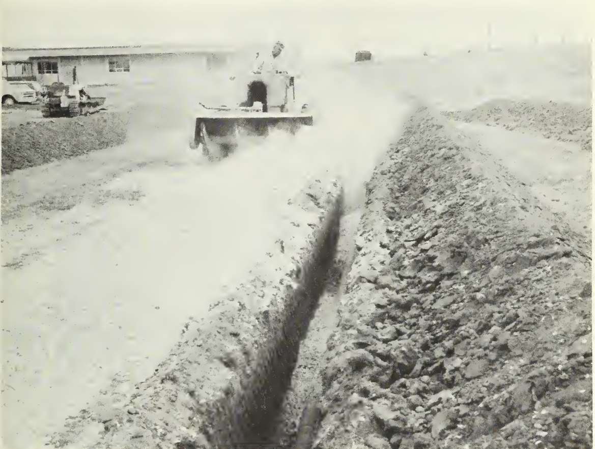
Organic blinding and filter materials (wood shavings). (Photo No. 0-2670-11)
