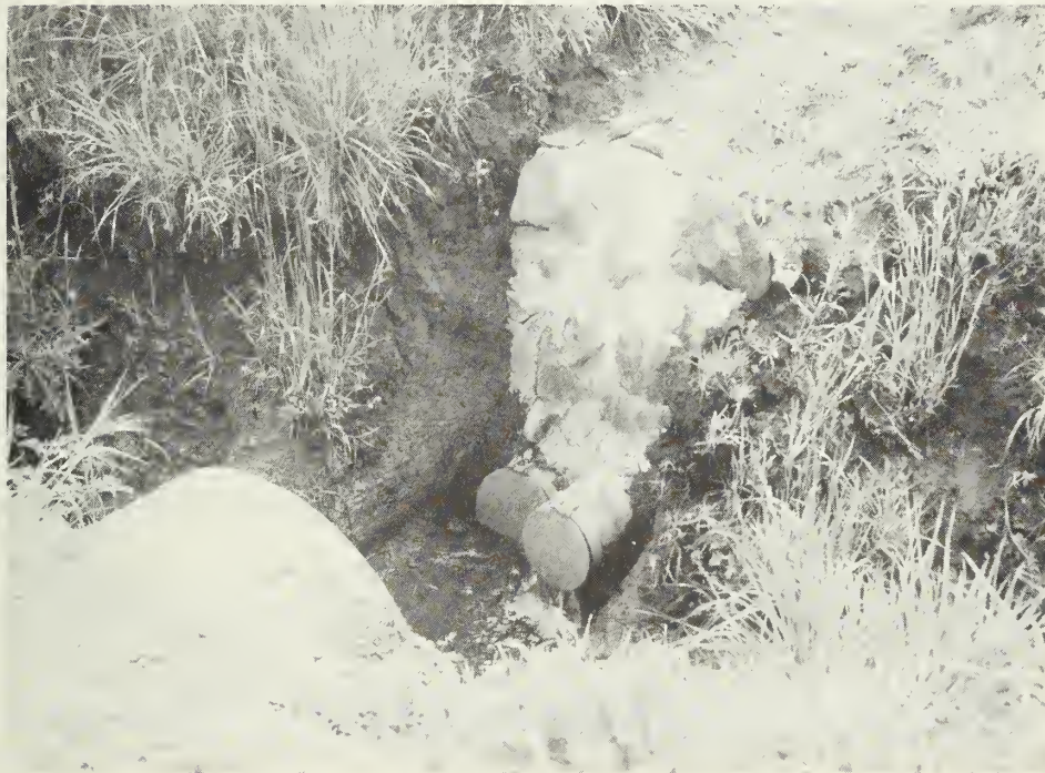
Outlets for two tile drain lines protected by flap gates to prevent entry of rodents. (Photo No. 0-1251-12)
