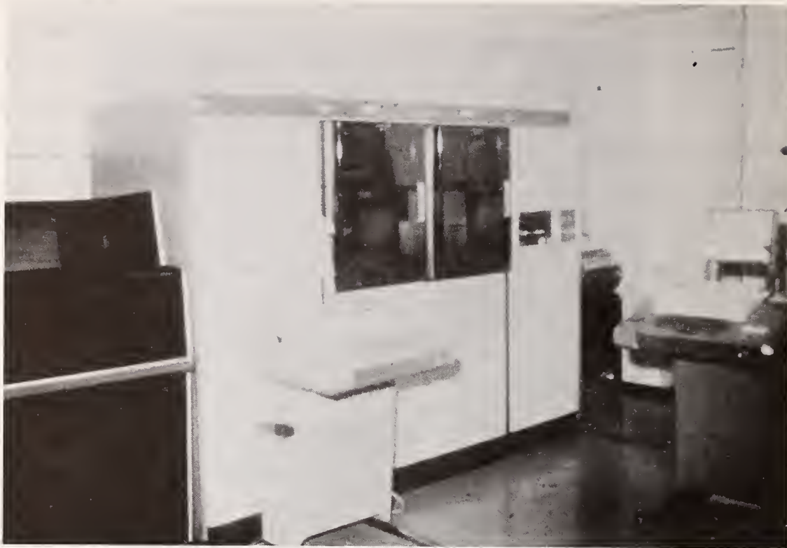
FIGURE 5-10: COMPUTER SYSTEM USED TO CONTROL HADDONFIELD. Left to right: printer, disc cabinet, two tape units, mini-computer, card reader, and two TTY's in foreground
