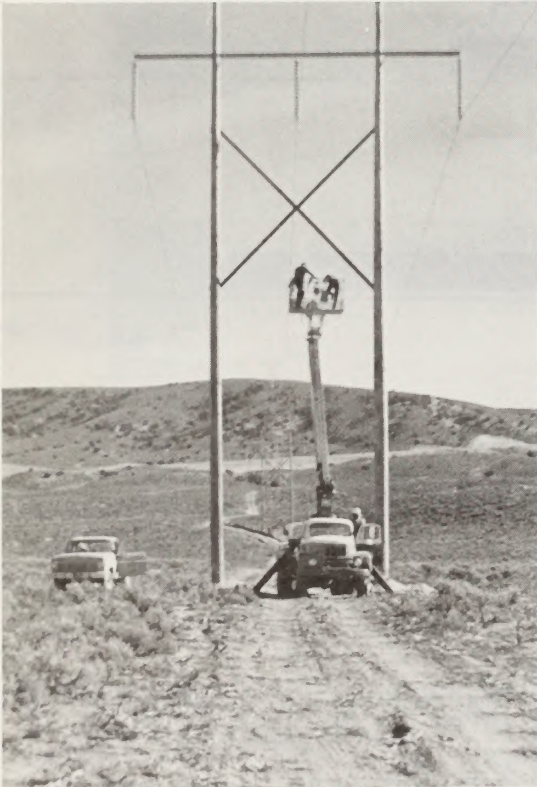
Typical disturbance resulting from transmission line construction in northern Nevada. Cross-braced H-frame towers traversing northern desert shrub type. (Sigurd, Utah to Ft. Churchill, Nevada 230 kv transmission line.)
