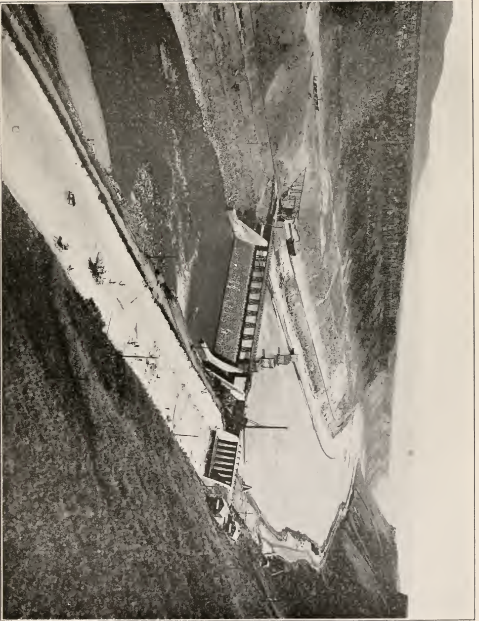
BOISE DAM AT WHICH THE RECLAMATION SERVICE IS NOW ERECTING A POWER PLANT, THE POWER TO BE TRANSMITTED TO AND UTILIZED IN THE CONSTRUCTION OF THE ARROWROCK DAM.
