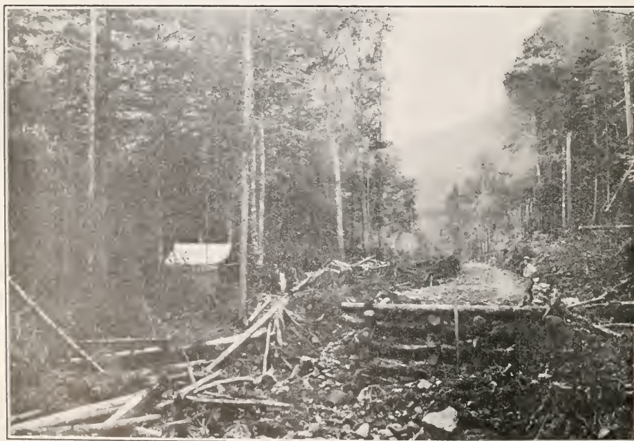
GRADED LOGGING ROAD; GRADING COST $16 PER MILE. FOUNDATION FOR TRESTLE IN FOREGROUND. NEW EXTENSION OF LOGGING RAILROAD THROUGH FRANCONIA, N. H.
