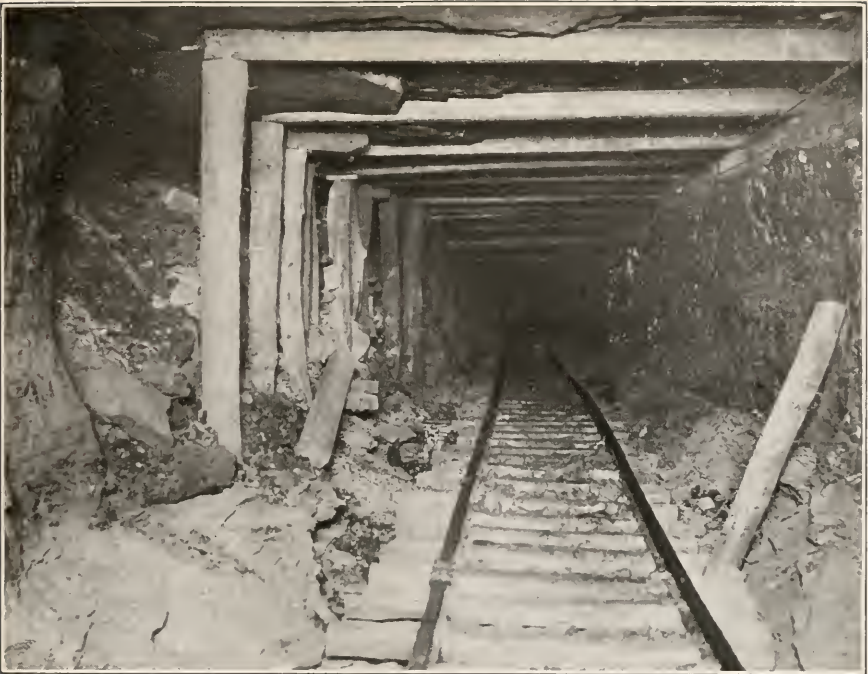
PLATE I. STEEL ROOF SUPPORTS RESTING ON TIMBERS IN BARTON MINE, THE MIDDLE STAGE, HALF TIMBER, HALF STEEL.
