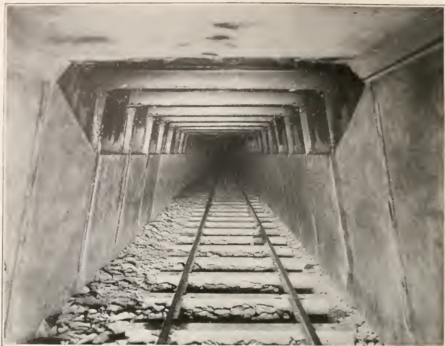
PLATE III. STEEL GAUGEWAY SUPPORTS IN EN- TRANCE TO ALLPORT MINE. ALL STEEL AND CONCRETE
