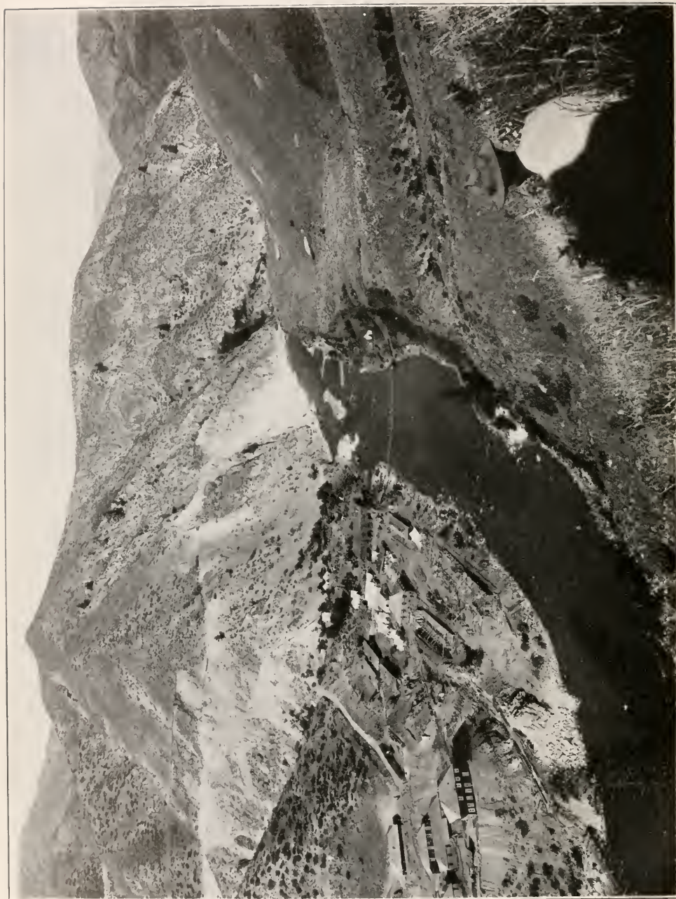
ARROWROCK DAMSITE AND GOVERNMENT CAMP. THE EXCAVATION ON THE LEFT IS FOR A ROADWAY AND MARKS THE LINE OF THE TOP OF THE DAM.
