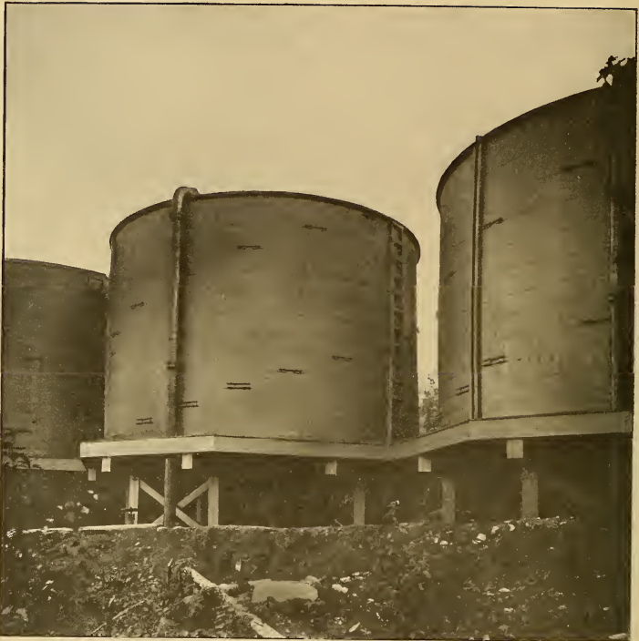
FIG. 11.—THE HOTEL MT. WASHINGTON STORAGE TANKS, EACH OF 50,000 GALLONS CAPACITY
