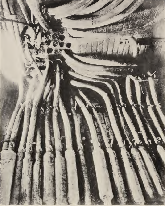
FIG. 43.— Underground cables in a manhole
