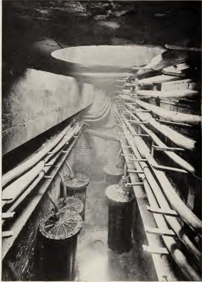
FIG. 47.— Loading-coil pots in a manhole
