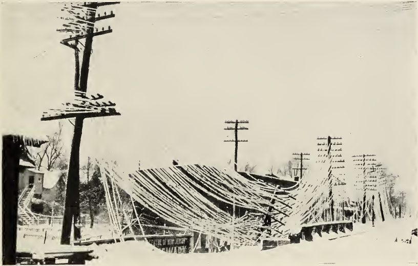
FIG. 58.— Damage caused by wind and sleet
