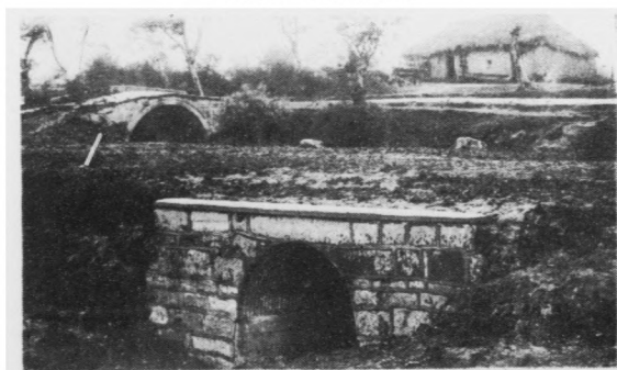
上：安徽段內半圓綑紋鐵管涵洞 Above—A Semi-circular Corrugated Steel Culvert—Anhui Section
