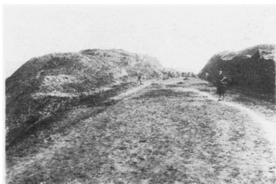
程工山開近附城宣內段徽安：上 Above—Rock Excavation near Suncheng —Anhwei Section
