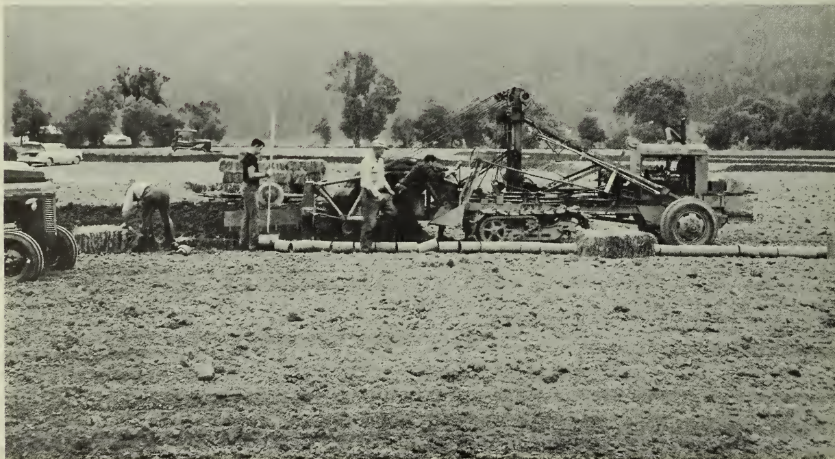
Photo 30.--Some fields are drained by a pattern-type tile system, Clatskanie Soil Conservation District, Oregon. SCS photo
