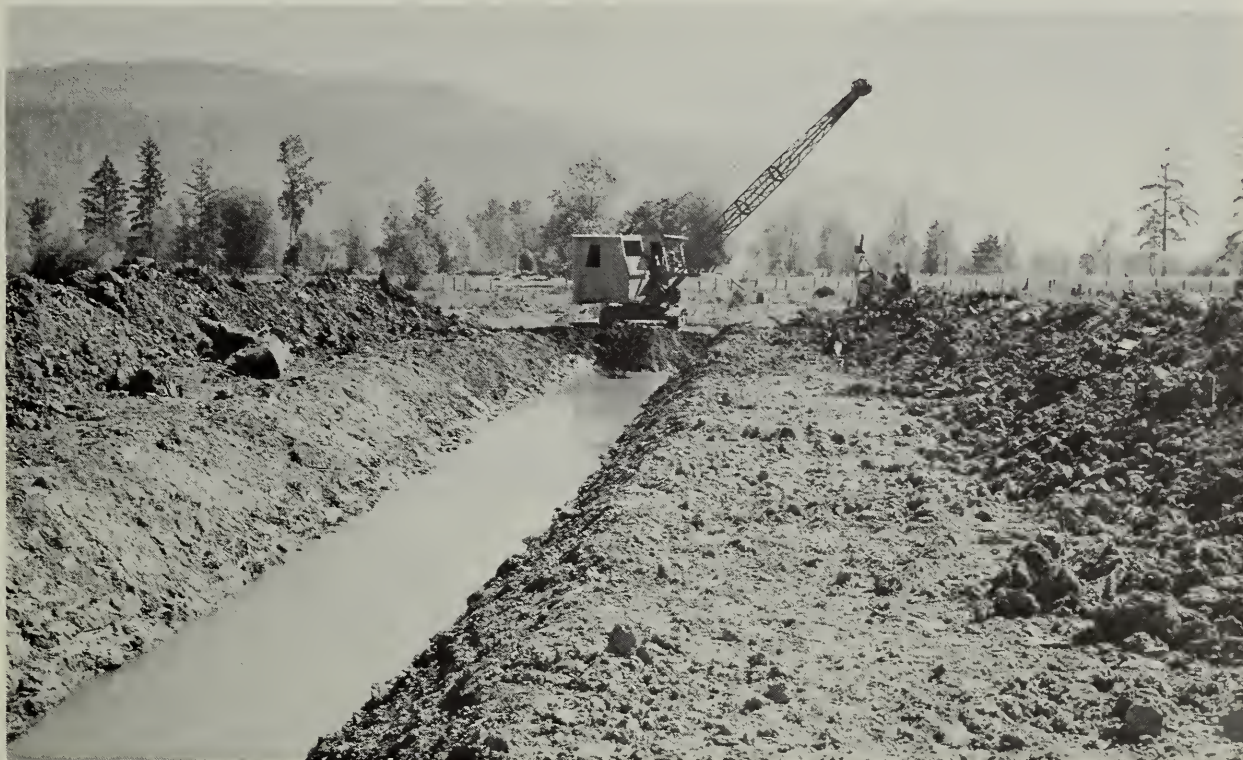
Photo 31.--Often tile cannot be used successfully to drain land until outlet ditches have been built, Tillamook County, Oregon. SCS photo
