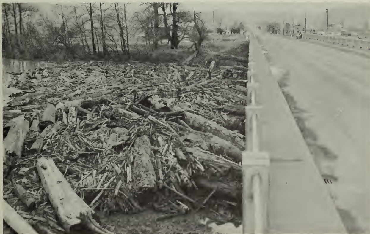
Photo 27.--Debris against U. S. Highway 101 bridge must be removed before the bridge is damaged, Trask River, Oregon, 1956. SCS photo.
