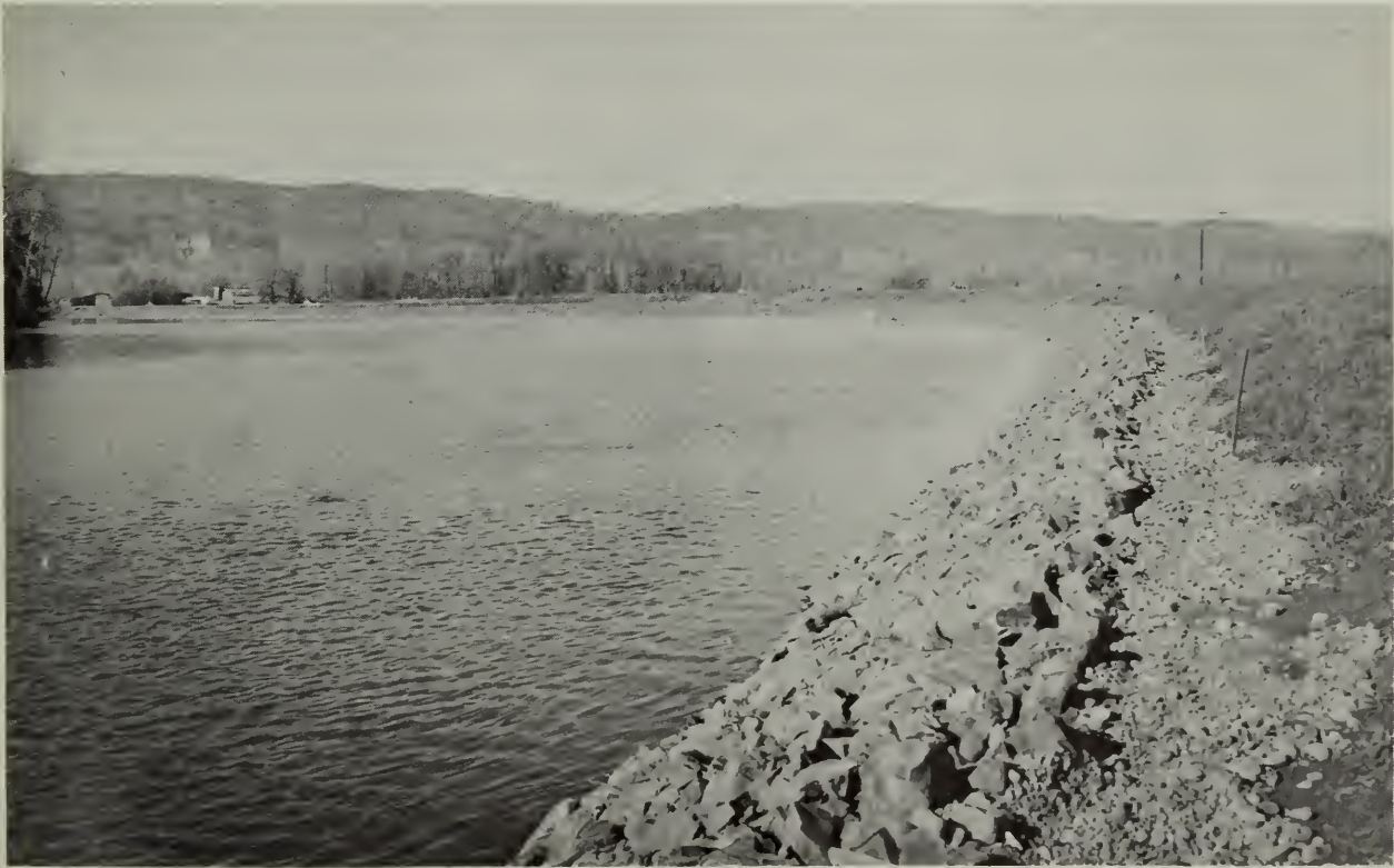
Photo 29.--This portion of the Clatskanie River bank has been protected by rock riprap, Oregon, 1962. SCS photo
