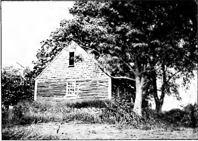
Interesting from without, but what of the internal conditions? If it can be saved, it is worth while, as its setting is unique and hard to duplicate
