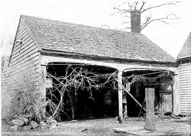
An open woodshed with good, simple details, giving a large area of openings. Its attachment to the house is bad, however
