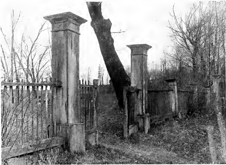
There is no elaborate treatment to this fence, but it suggests being put there with a purpose. There is a stone base or foundation below the wood fence sill
