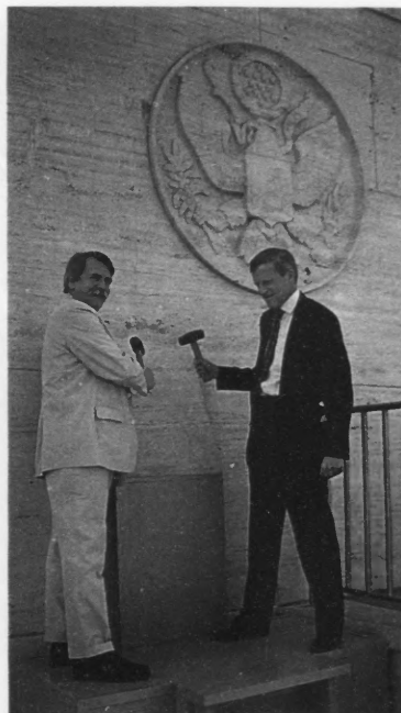
HAVANA, Cuba—Foreign Buildings Operations' Joseph Toussant, left, and principal officer Joseph Sullivan begin renovation of the U.S. interests office building.
