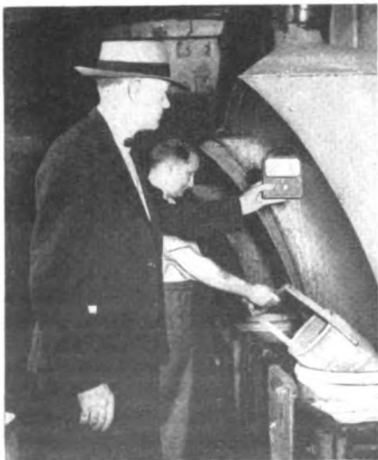
An industrial hygiene engineer measures the rate of air movement into the hood. Exhaust ventilation protects the worker from the fumes of the acid into which he is dipping metal parts.
