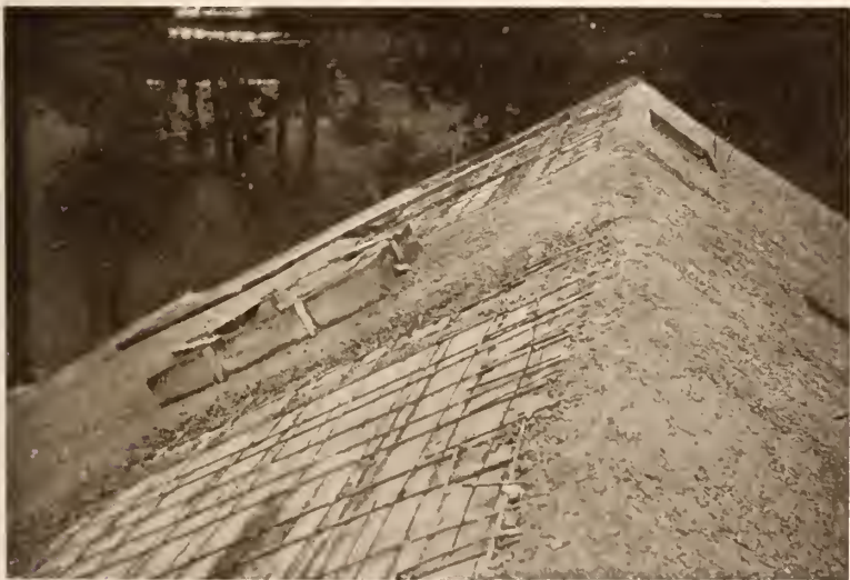
8—The Roof, its First Coat of Concrete and the Reinforcing Rods in Place
