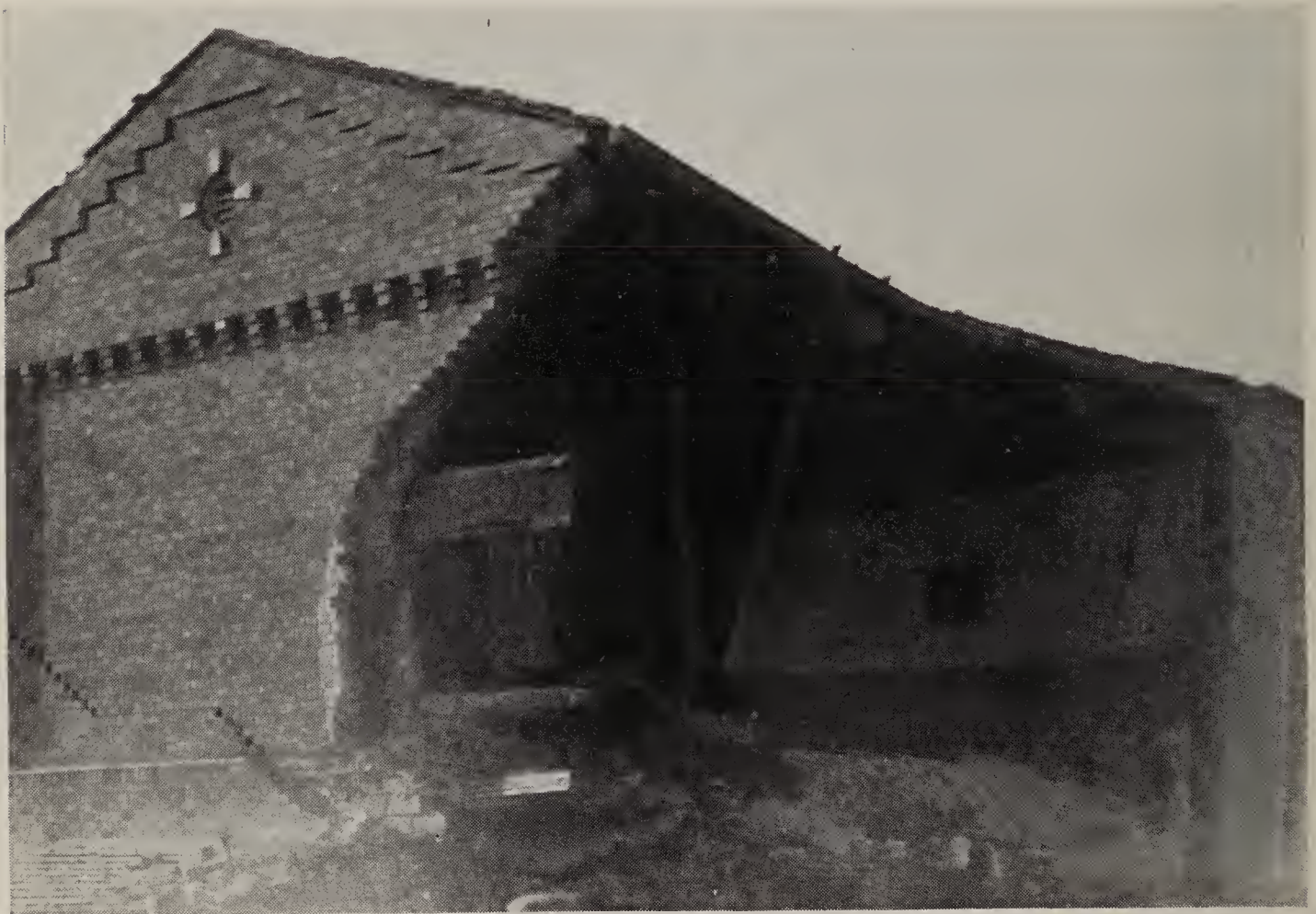
Close-up view of second floor of graded school at southeast corner of building.
