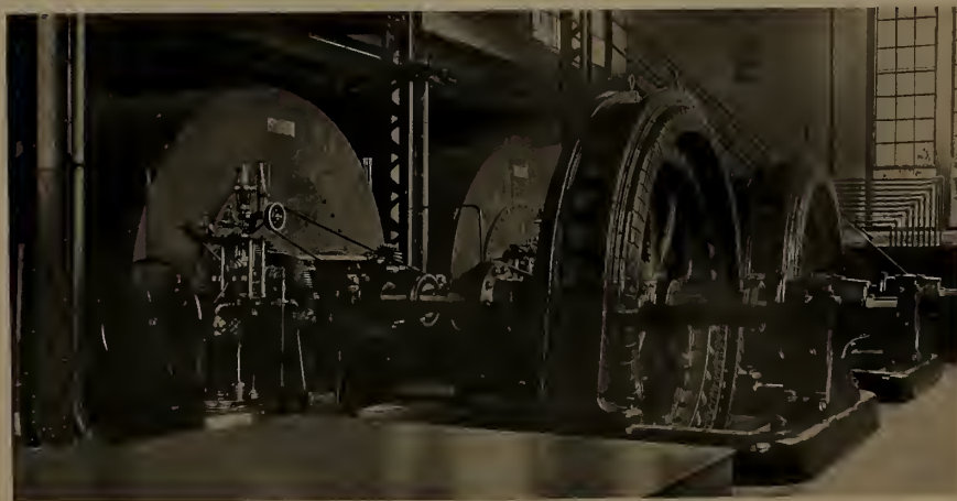
TWO 1100 H. P. McCORMICK HOLYOKE TURBINES IN HOLYOKE WATER POWER CO. POWER PLANT
