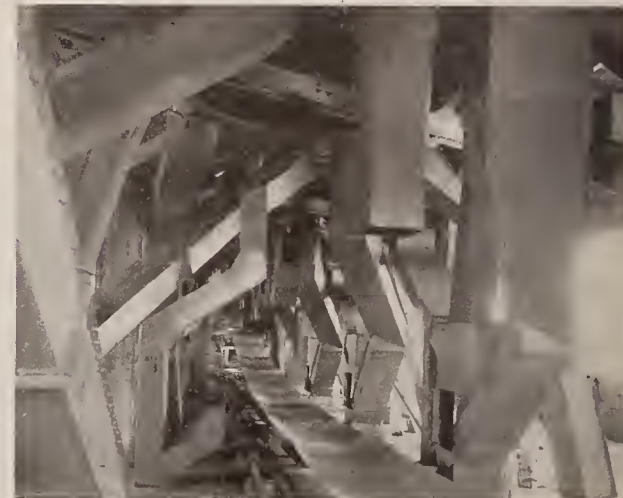
DISTRIBUTING SPOUTS UNDER SCALE FLOOR
