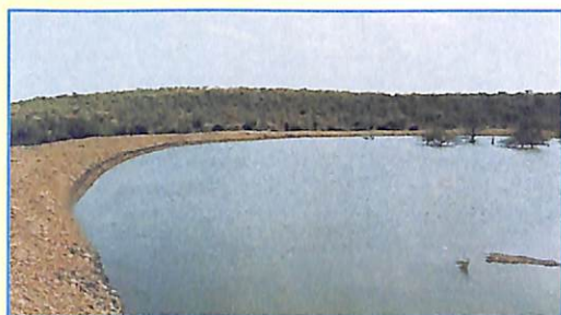
Based on the decisions of Gram-Sabha, construction of RWH Structures in the village gets start
