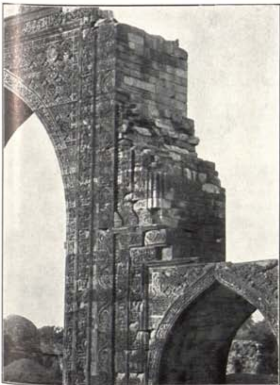
(c) QUTBU-D-DIN'S ORIGINAL SCREEN. DETAIL VIEW OF BROKEN JAMB OF UPPER SUBSIDIARY ARCHED OPENINGS (NOW MISSING). SEE DRAWING IN PLATE No. IV FOR RESTORATION OF SCREEN.
