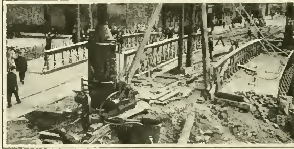
The bridge was cut in two parts and while one half was being repaired the other half was being used by cars
