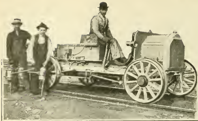
Driving spikes in railroad ties is accomplished with socket-wrenches run by motor
