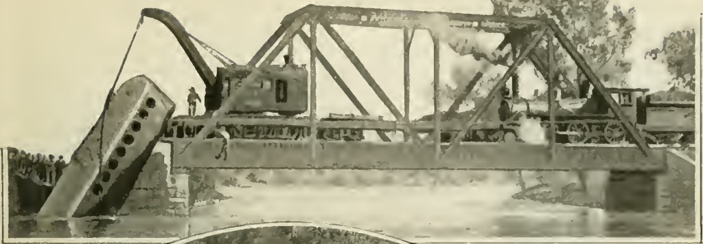
Above, the crane has its "hands full," but fortunately for it the car is of steel and can stand the heaviest pull
