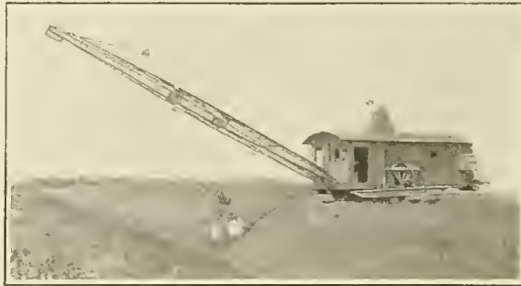
This excavator is being used with success by the United States Government on one of the great irrigation projects of the arid Southwest
