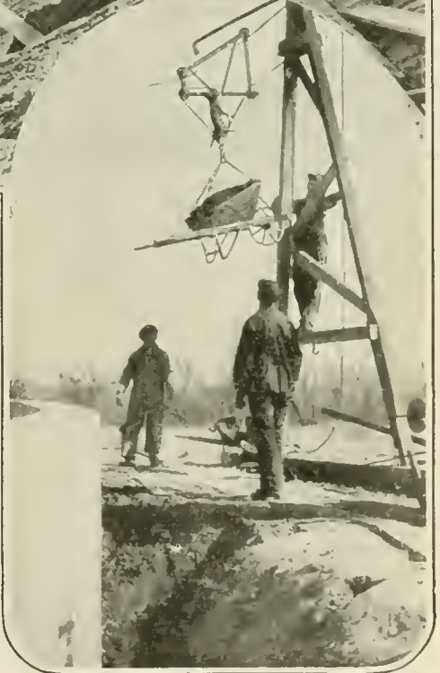
Releasing the Hoisting Line at the "Two-Block" Position Lowered the Wheel-Barrow
