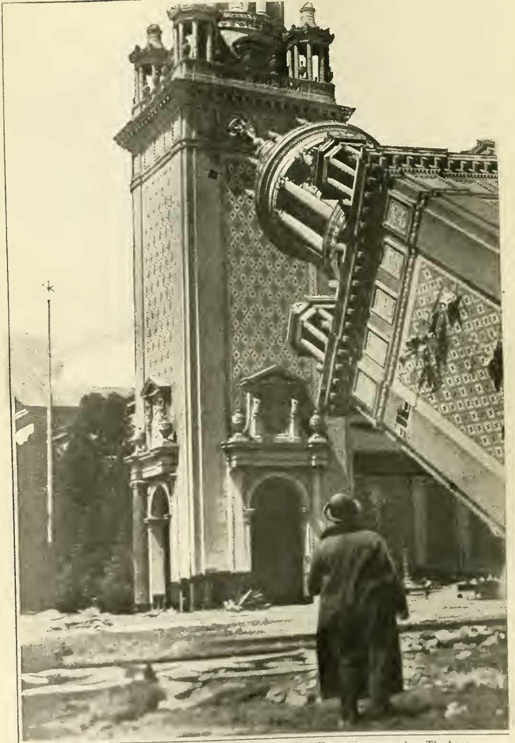
Wrecking the Italian Towers at the Panama Pacific Exposition grounds. The base
