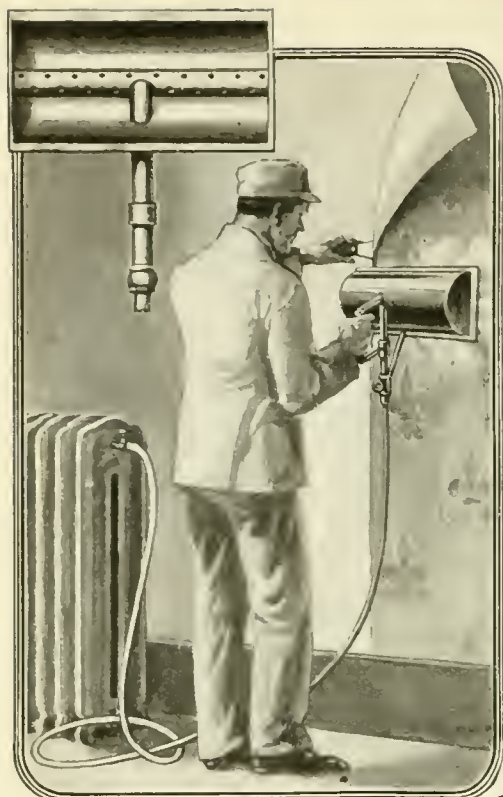
A nearby radiator supplies the steam through a hose to the apparatus in use
