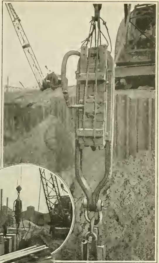
Piles can be drawn in less time than it takes to drive them with this inverted steam-hammer
