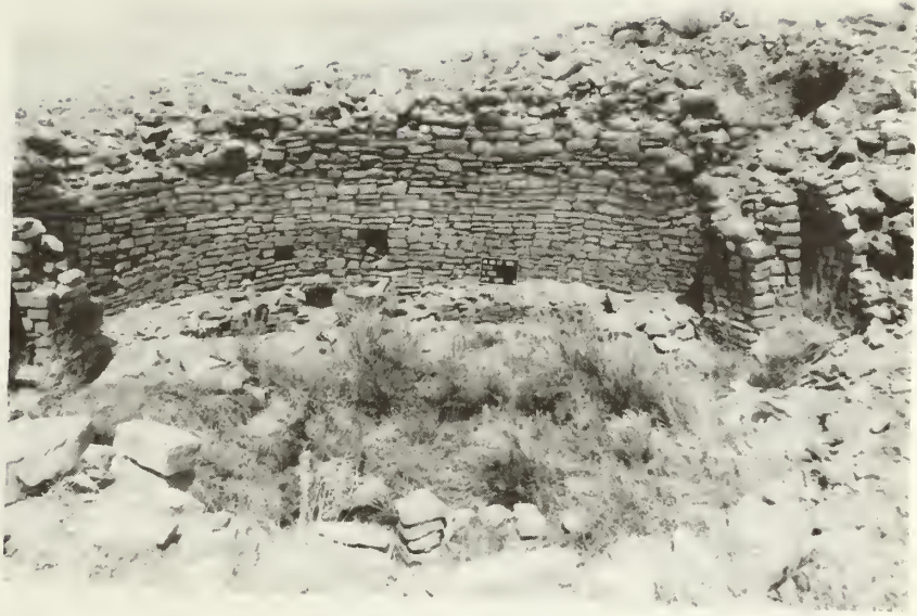
Kiva, north wall: before stabilization
