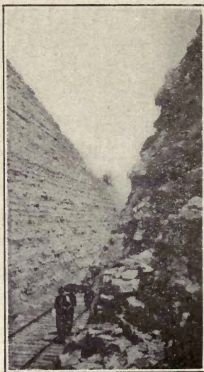
13. EDEN SHALE AND LIMESTONE Cut on Maysville-Paris Branch of the Louisville and Nashville Railroad, Nicholas County. Photograph by A. M. Miller
