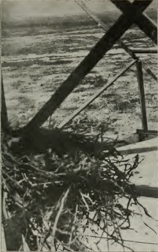
Young Raven's Nest in Electric Power Line Tower.
