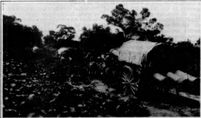
PHOTO FROM NORTHROP CLAREY, N. Y. C. Hauling 15-inch Casing Across Country Where the Wheels of the Carts Made Their Own Roads
