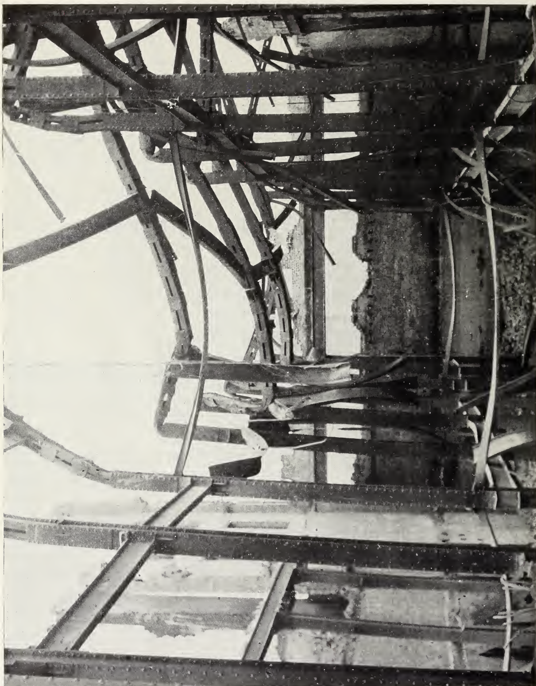
DESTROYED IRON FRAMEWORK, SAN FRANCISCO.
