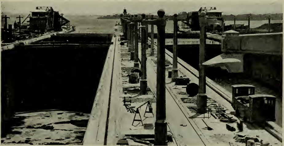
Lake end of Gatún locks looking out over Gatún Lake. Three different stages in filling the locks are shown, the lock at the left being empty, the one in the lower right-hand corner half full and the one in the upper right hand corner full. Emergency dams are seen in the background. Four locomotives similar to the one shown are to be used for each ship, two being in front and two in the rear
