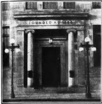
Limestone doorway with bronze doors showing the richness that can be added to the simple dignity of the stonework by this one touch of metallic refinement. Bound Brook, N. J.
