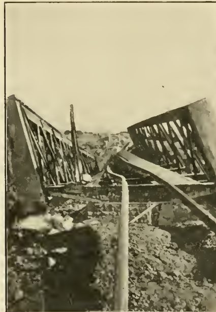
SHORE SPAN OF THE KROONSTAD BRIDGE WRECKED BY DYNAMITE.
