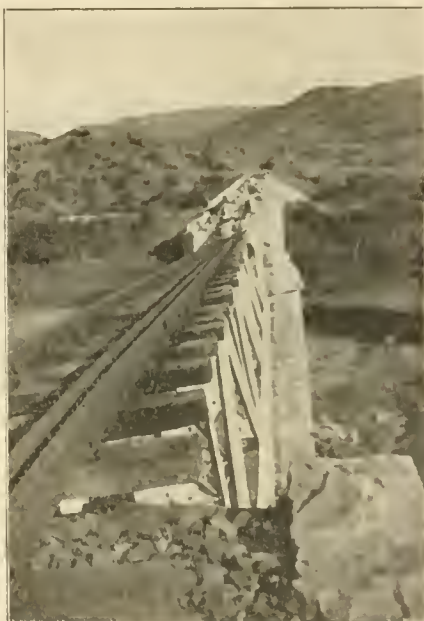
AVOCA BRIDGE FROM ABUTMENT AFTER EXPLOSION OF DYNAMITE.
