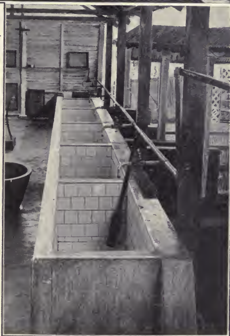
TWO VIEWS OF DILUTION AND MIXING TANKS.
