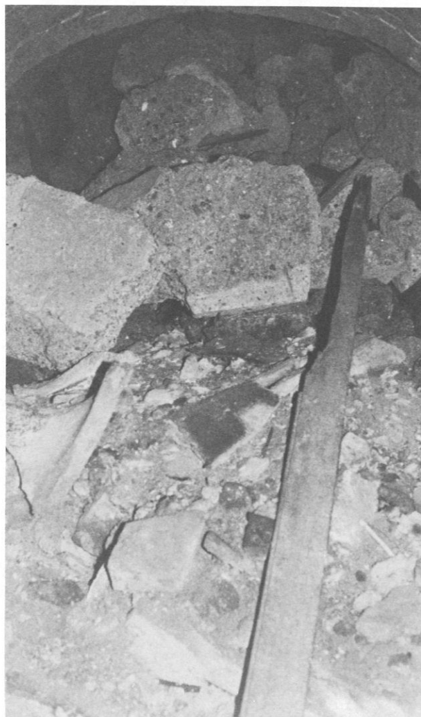
Rubble fills the tunnel beyond the wall.
