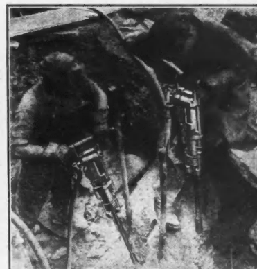
CP-10 Sinker Drills, Dry, team-working for the Brooklyn Edison Company, Brooklyn, N. Y.
