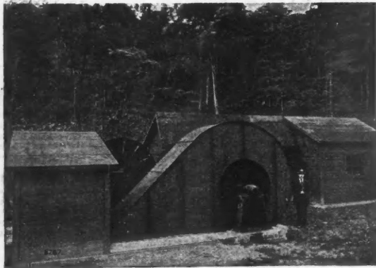
Double Inlet Blowing Fan installed at a shaft mine. Note displaced propeller type in back-ground. Capacity 100,000 cu. ft. at 3-in. water gauge.
