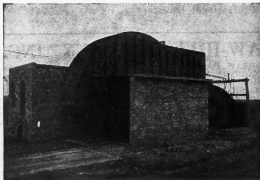
Double Inlet Primarily Blowing Reversible Fan installed at a shaft mine. Capacity 350,000 cu.ft. at 4-in. water gauge.
