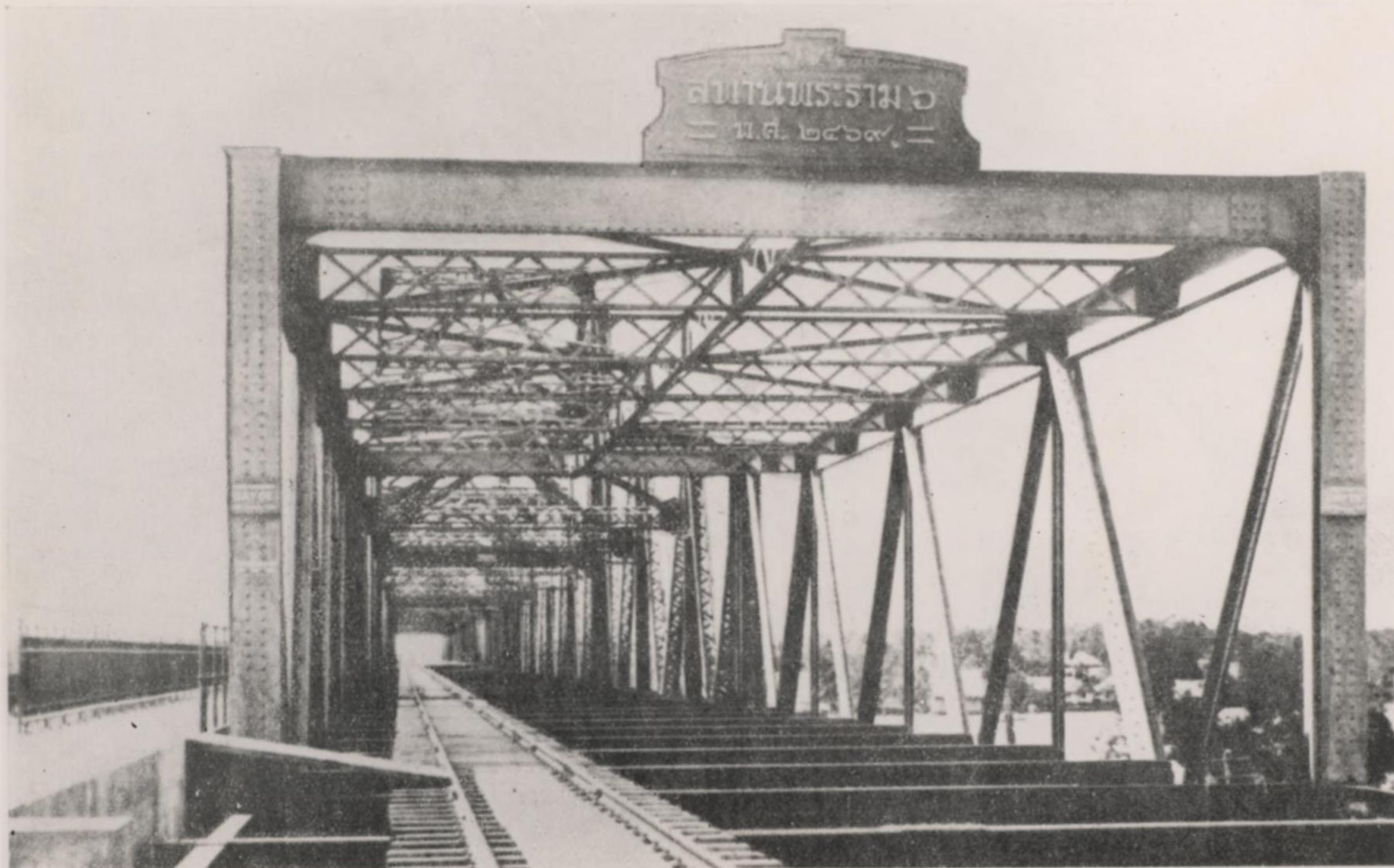
23. Rama VI Bridge during construction, showing cantilever footway on left, railway in centre, and space for future roadway on right
