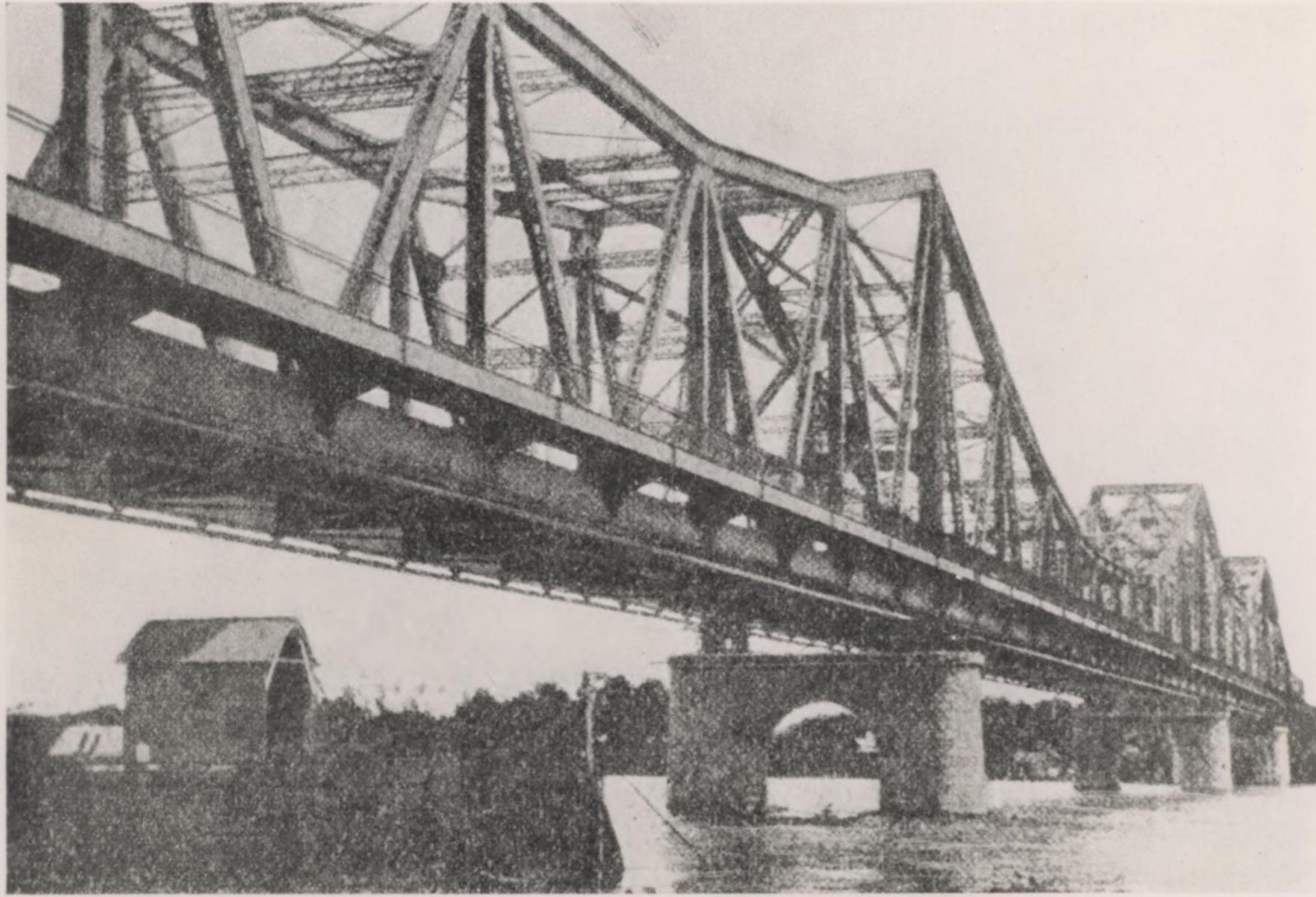
22. Rama VI Bridge from under one of the 84 metre spans. A 39 inch steel water-main is carried under the bridge, leading from the waterworks to the West Bank City
