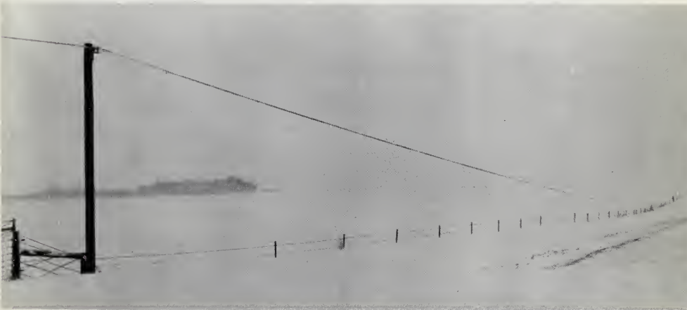
Long span wires on ground after storm.
