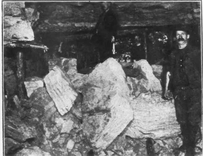
FIG. 2. SHOWING FALL OF HARD SANDSTONE COVER IN THE "CD AND EF" MINE
